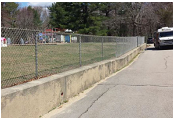
Before: Access to the outdoor play area posed safety and accessibility issues.
